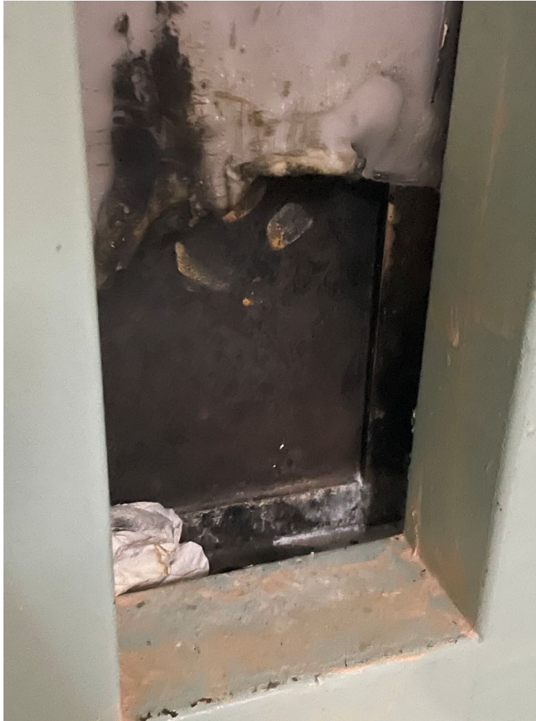
Cell Window in Komohana with metal plate covering and what appears to be melted plastic.
